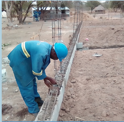
Construction of pavement beam structure in Madombatomba Primary School, in Chibabava, October 2020.
